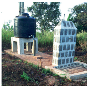
Storage Tank and Tap
