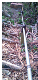
Self Installed Supply Pipe
